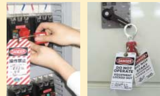
Lock-out and tag-out Example when multiple workers are at work
